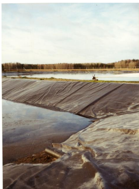
Figure 4. Rubber sealed dams for storage of blackwater. Example from Enköping, Sweden. Photo: Ebba af Petersens.
