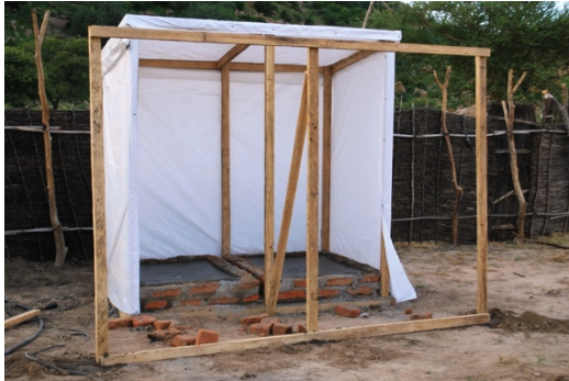
Cholera Treatment Center toilets / showers
